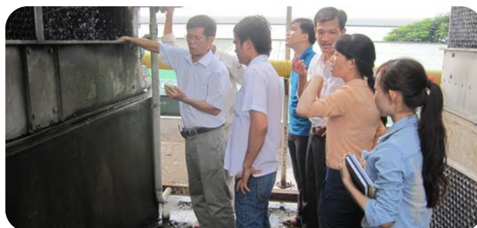
Photo: Instructing technical staffs to assess performance of condenser-compressor unit at A Chau factory.
