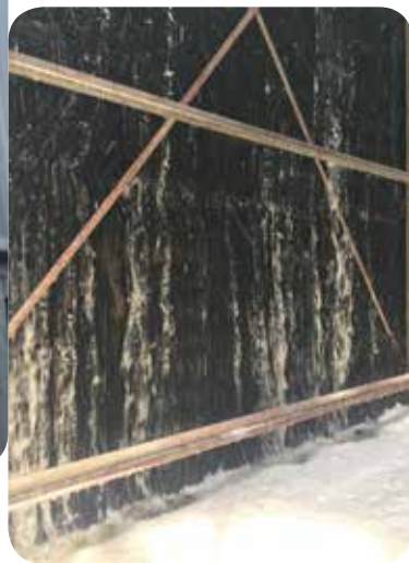
Uneven distribution of cooling water in the condenser
