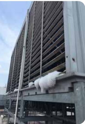
Poor maintenance of condenser causing bubbles
