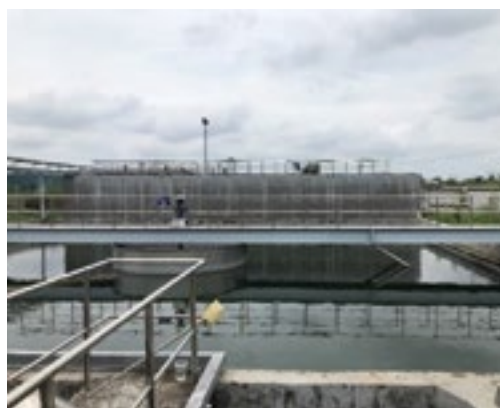
Common effluent treatment plant of Xuyen A IP
