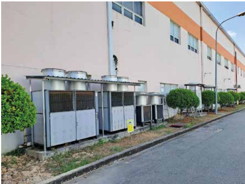
Energy-saving solutions implemented for air conditioners
