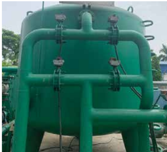
Existing wastewater recycling tank
